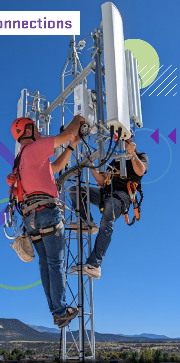
UEN Field Engineers Scott Larsen and Brad Morris install radios that supply connectivity to a school in rural Beaver County School District.
